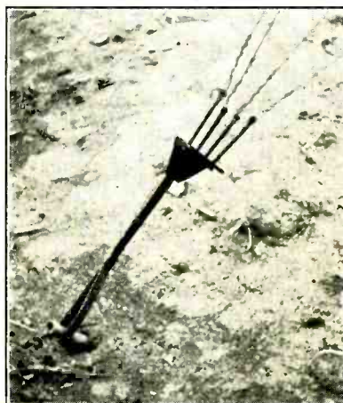
Showing how the guys for one direction all terminate at the same point. The gadget shown is the equivalent of separate turnbuckles in each of the four guys.
